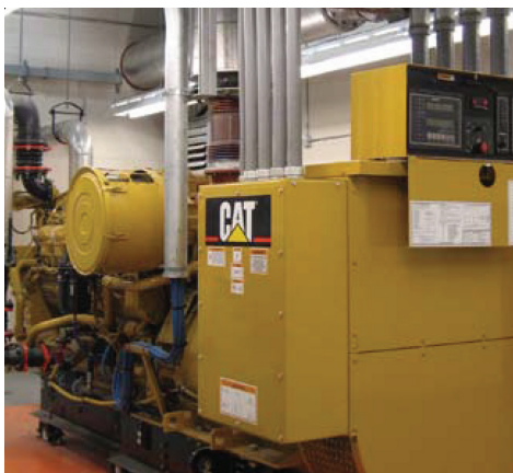
One of two Cat® 3512B 1500 kW standby generators.
